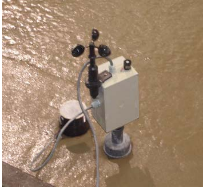
Figure 3 On-site CMS Setup.
